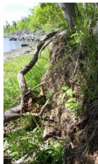
Photo 10: Eroding Coast North of the Causeway
